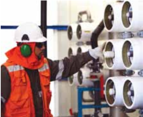
Osmosis plant at El Tesoro.
